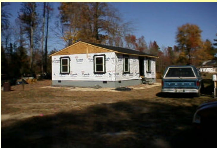
A house under construction by Gloucester Housing Partnership as part of the Indian Road project. Students in the Partnership's training program are helping build the new house, which will replace a nearby trailer.
