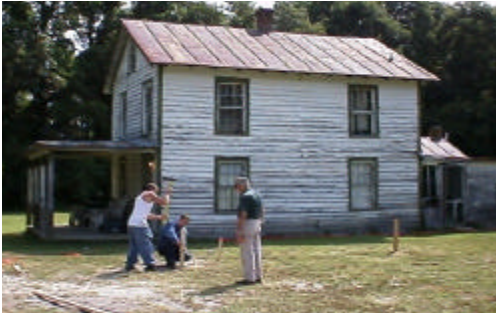
The apprentices of GHP layout the foundation of Mr. Ward's new home.
